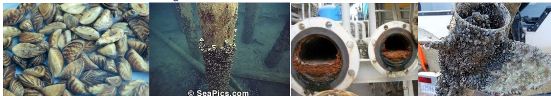
Figure 40: Zebra Mussels & Damages
